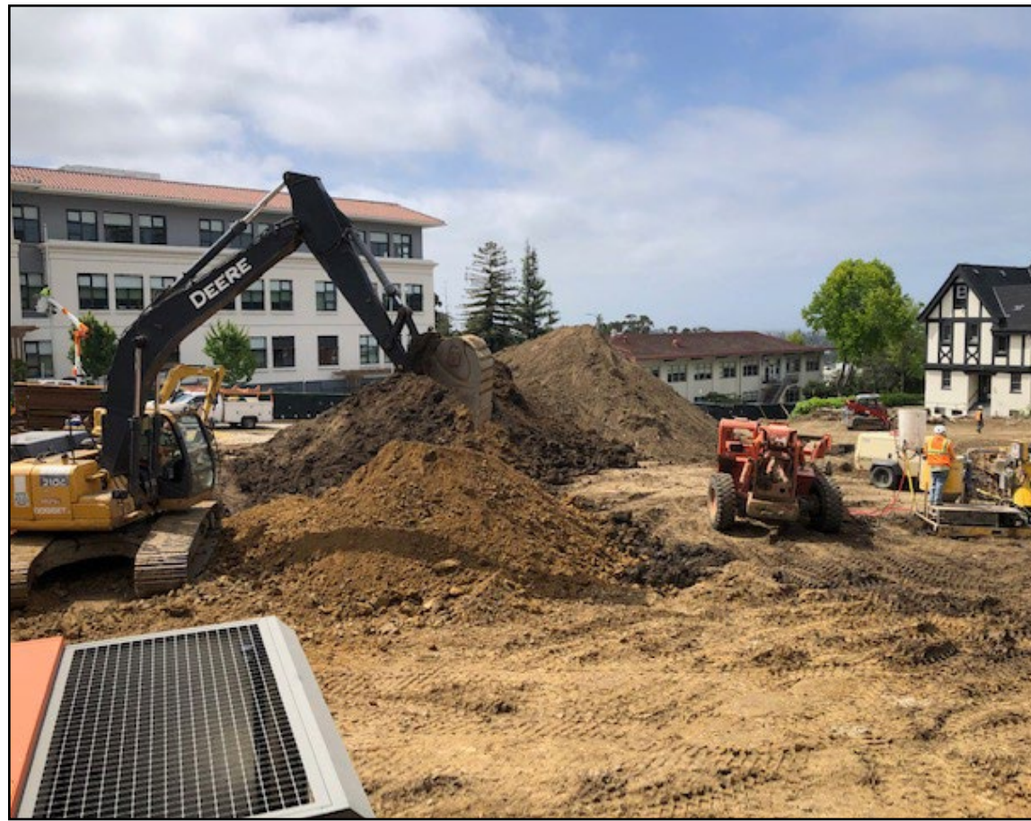
Soil is piled to be hauled off from the community pool site.
