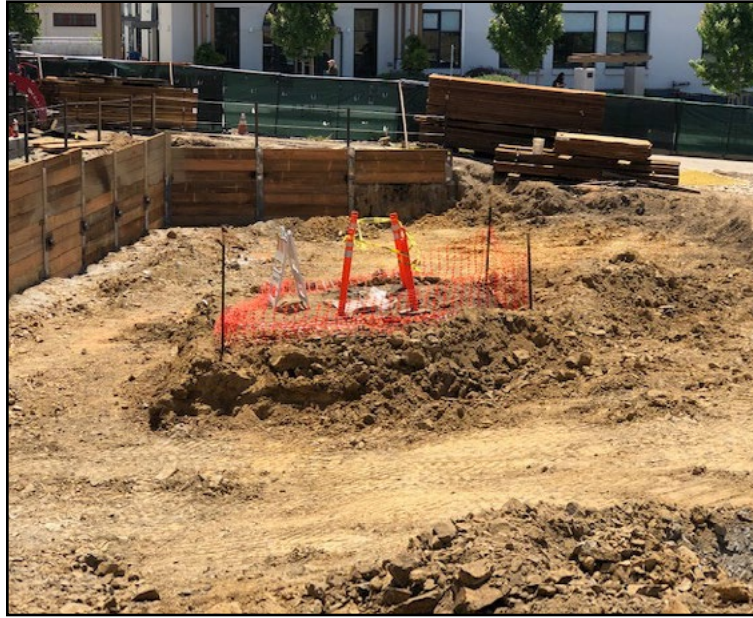
Orange posts and nets section off the area where a century-old fuel tank, still containing gasoline, was found buried at the pool site.
